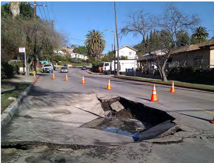
Figure 4-48. Subsidence example in San Joaquin Valley.
