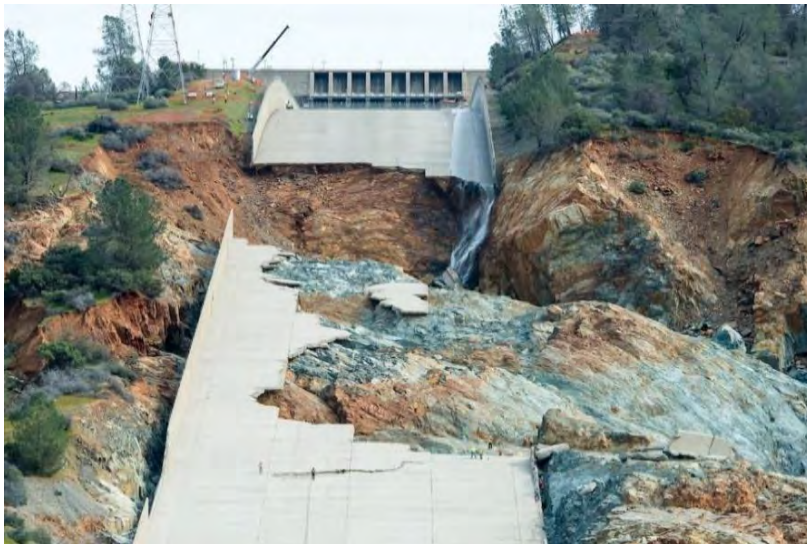
Figure 4-23. Oroville Dam Spillway after 2017 failure.
