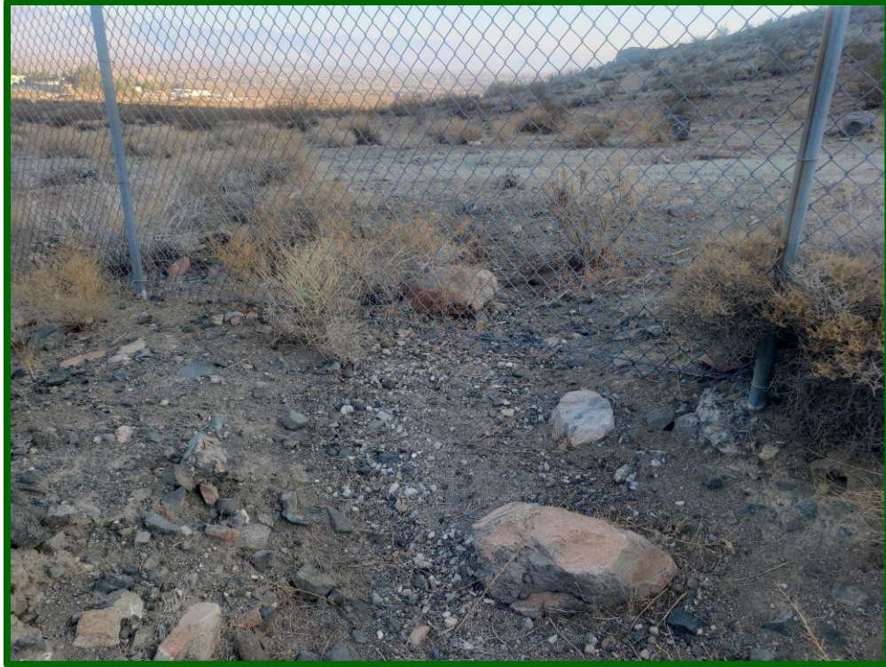
Exhibit 9. College Site: Gap under the north side of the perimeter fence.
